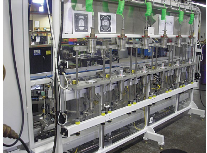
This six-station, hard-vacuum system was built to check lithium-ion batteries for leaks. Photo courtesy Vacuum Instrument Corp.
